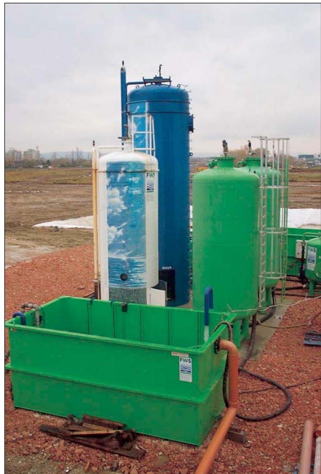
Water is pumped for the sedimentation basins, 400 m 3 , into a higher located basin to build a potential gradient. Afterwards the water runs through filter and adsorption units.
