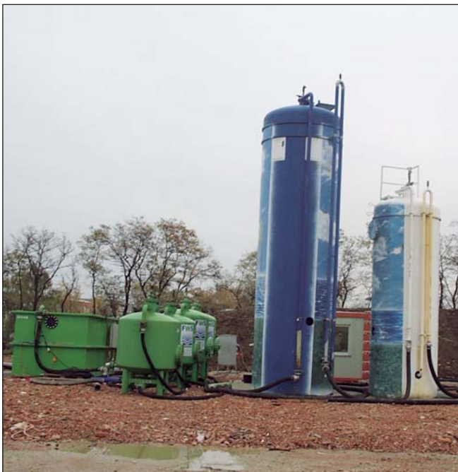
First the water runs through gravel filters (front), then through liquid phase activated carbon filters (back). All plant filters are equipped with connections for backwashing.
