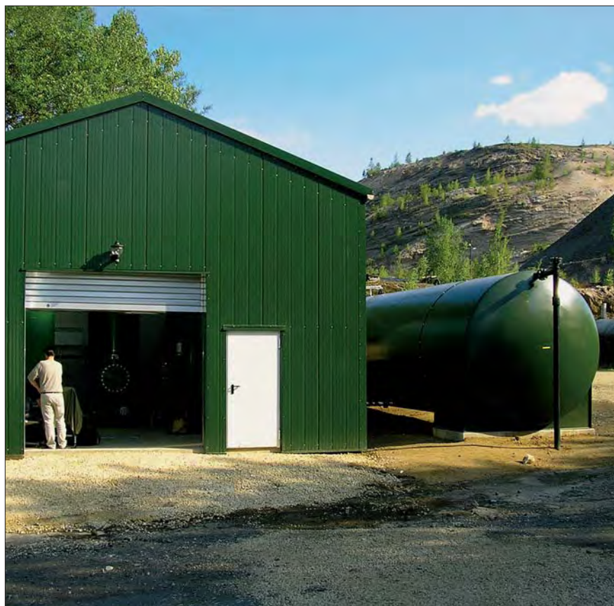
A 80 m 3 water tank compensates for variations in the leachate quantity. In the tank, the liquid level is measured continuously. Based on these measurements the flow rate to the treatment plant is controlled.
