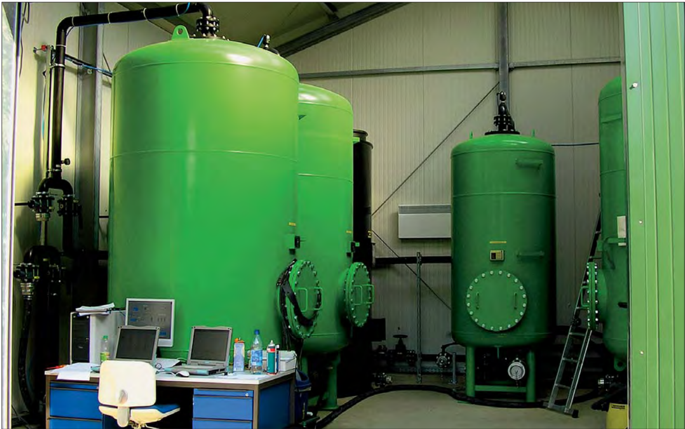
The treatment plant is controlled by a PLC system.
