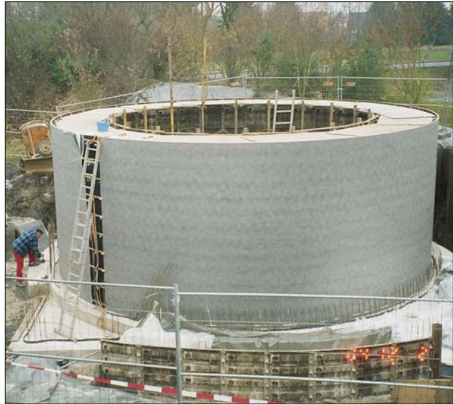
The storm overflow basin is a round container with a diameter of 10 m and a volume of 250 m 3 . For the construction of the container walls a special drain course was used.
