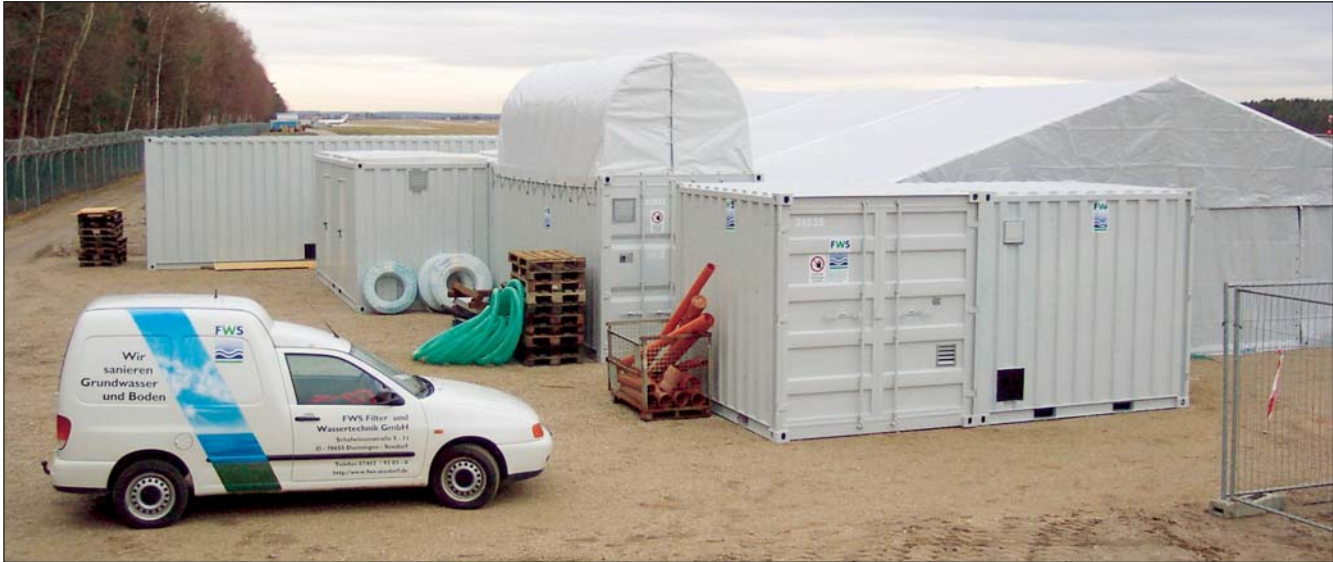
The groundwater and soil vapour remediation plant is designed for three remediation phases in dependence on the fade of contaminants.
