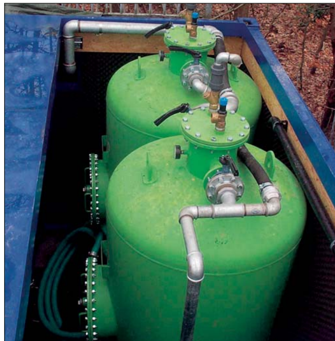
State-of-the-art treatment for the produced off gas is vapour phase activated carbon adsorption. BAUER Environment Group is developing a process modification to enhance the economic operation of the process treatment.
