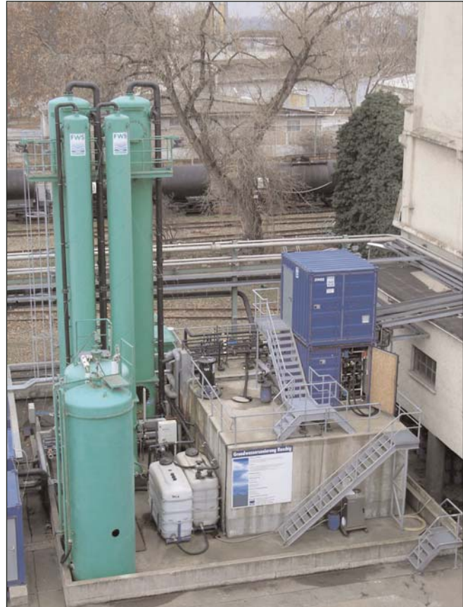
Contaminant removal adds to 120,000 kg considering the main contaminants Dichloromethane, Monochlorobenzene, Naphthalene, BTEX, VOC's. Additionally 48,000 kg free phase was recovered.
