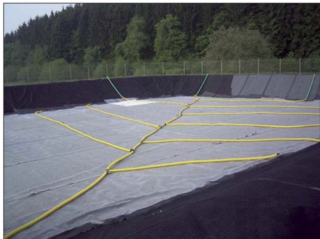
A protection fleece and a HD-PE foil serve as a base sealing. The drainage system is incorporated into a layer of coarse-grained lava.
