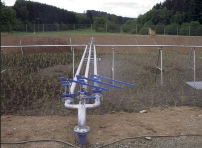
Filling system with high-grade steel pipes on support stands, forged pipe with ventilation valve and wedge gate valve.
