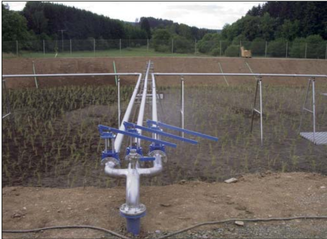
Filling system with high-grade steel pipes on support stands, forged pipe with ventilation valve and wedge gate valve.
