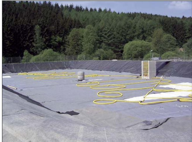
The drainage system for ventilation and drainage of sewage sludge has to be installed carefully to avoid damage of the sealing foil.
