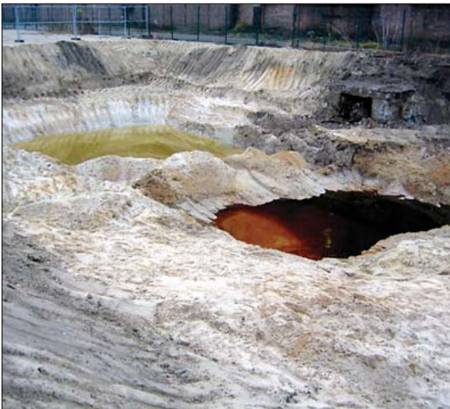
As the ground consisted of fine sands, it was possible to find remediated zones free from any contamination immediately adjacent to floating nonaqueous-phase liquid in the same excavation pit.
