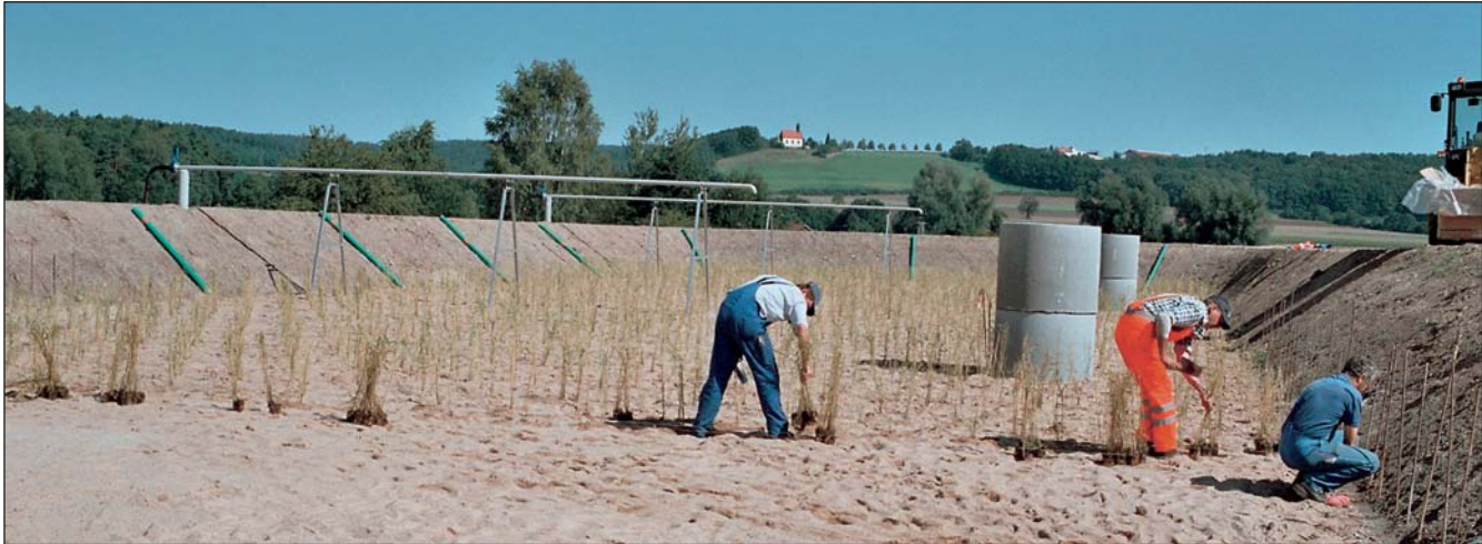
Implanting the reed plants into the patch. In the background two pipes on support stands made of high-grade steel and two controllable floor drains System PURE.
