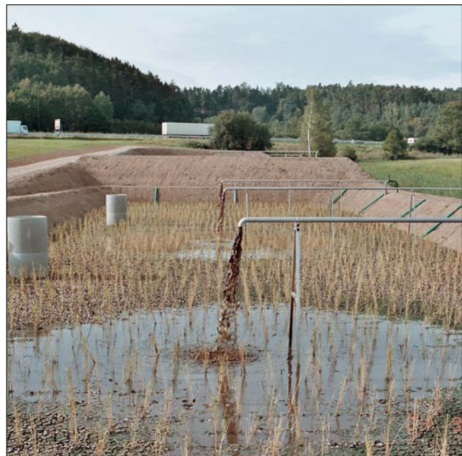
Patch 2 is fed with sewage sludge. The entire patch surface is already covered with highly drained sewage sludge, covered by cracks from drying. The treatment patch is close to the motorway A3.
