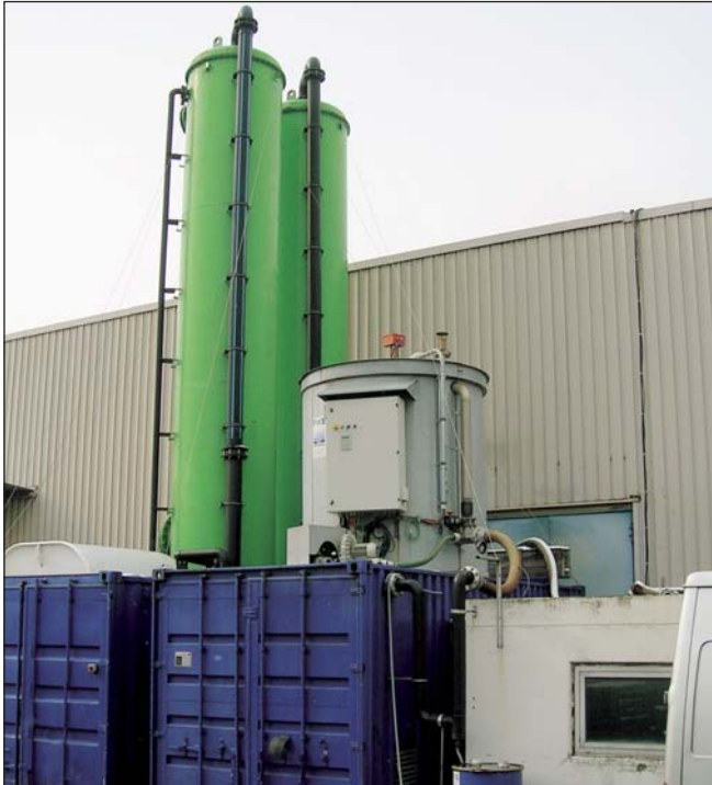
The picture of the treatment plant is dominated by the two 10 m high stripper towers. Catalytic oxidation takes place in a high grade steel container.
