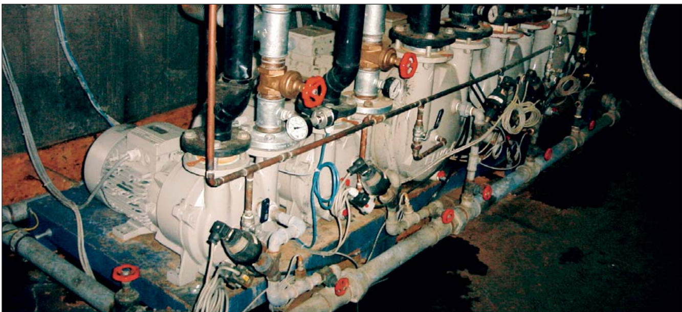
Two "water ring vacuum pumps" (WRVP) suck the soil vapour and transfer it to the catalytic oxidation unit. Three other pumps produce the necessary partial vacuum in the stripper towers.
