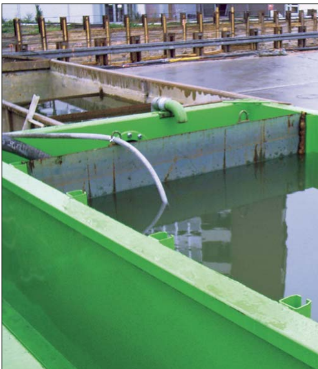
Treated water is discharged into the rain water channel or into the combined sewage channel.
