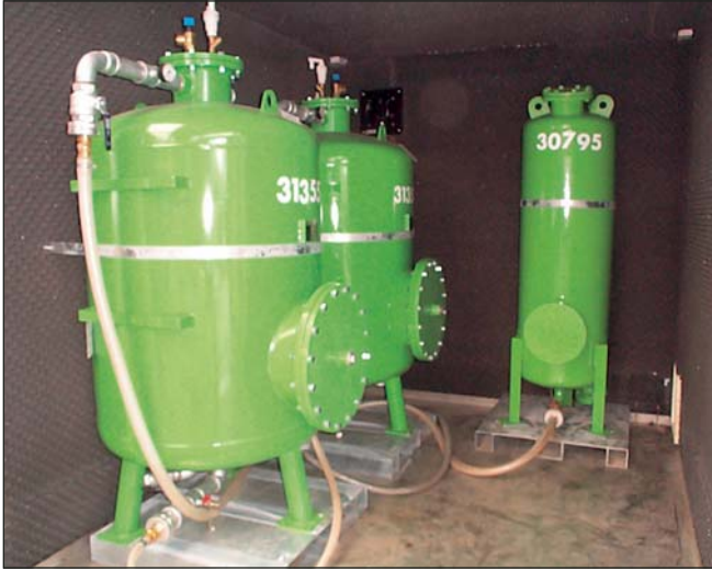
Remediation plant for dissolved pollutants installed in a common freight container with a capacity of 5 m 3 /h.
