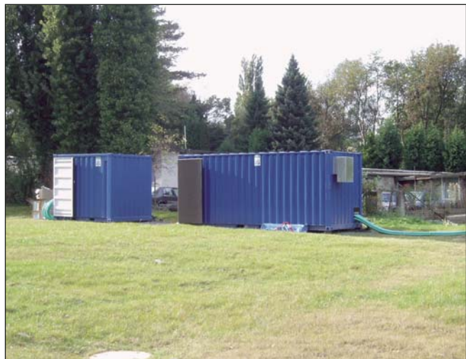
The soil vapour recovery system contains five drainage pipes, each is installed in parallel mode. Air-permeable granulates recover predominantly volatile substances.
