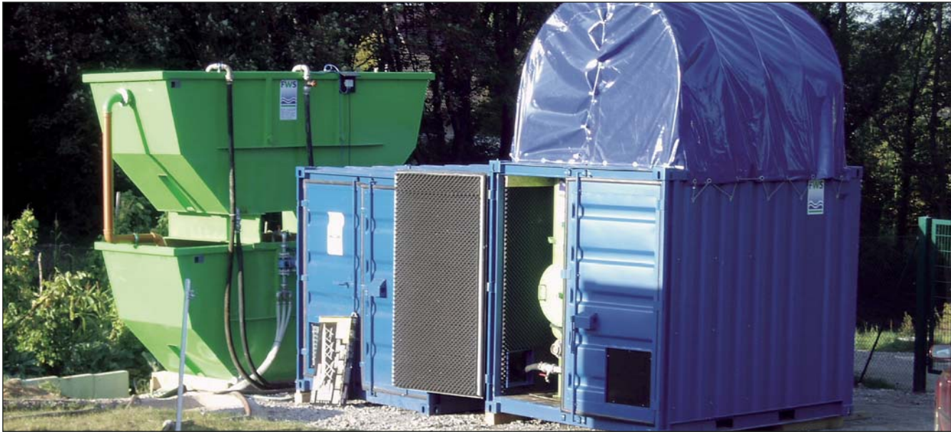
The groundwater treatment unit consists of a pure water and a back washing basin as well as a gravel and an activated carbon filter. Contaminated groundwater is recovered from approx. 20 m depth. Groundwater contamination was found between 10,000 µg/l and 100,000 µg/l for aromatic hydrocarbons and between 1,000 µg/l and 10,000 µg/l for halogenated hydrocarbon.
