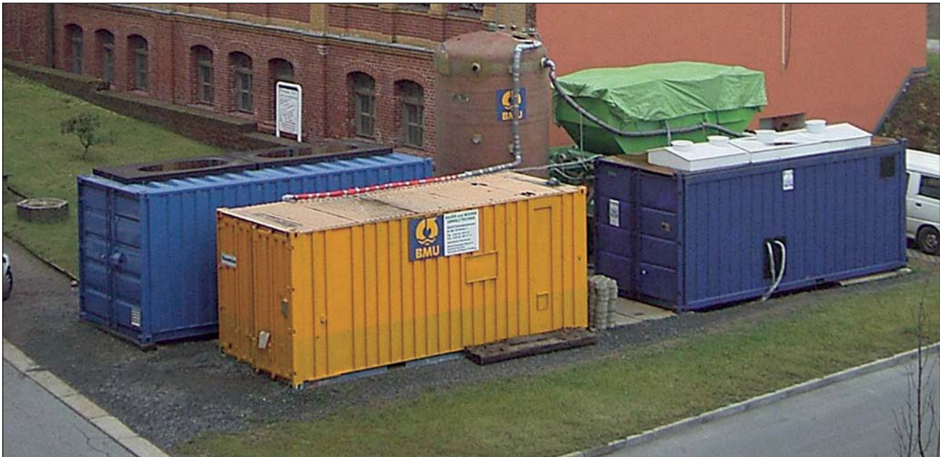
The treatment plant for chrome and halogenated VOC-contaminated groundwater is located in the midst of the revitalised industrial site. The components for the individual process stages are accommodated in the containers.
