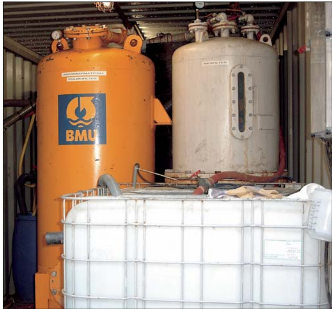
The plant consists of a chromate reduction, a precipitation and flocculation, a sedimentation and a filtration stage. Treatment of halogenated VOC's is achieved in liquid phase activated carbon filters.
