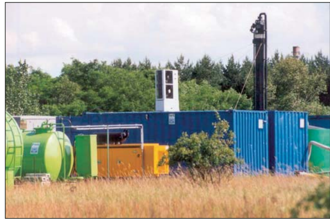
The Groundwater treatment plant is equipped with a kerosene storage tank, a power generator, a catalytic oxidation unit for off gas and a stripper for condensate treatment.
