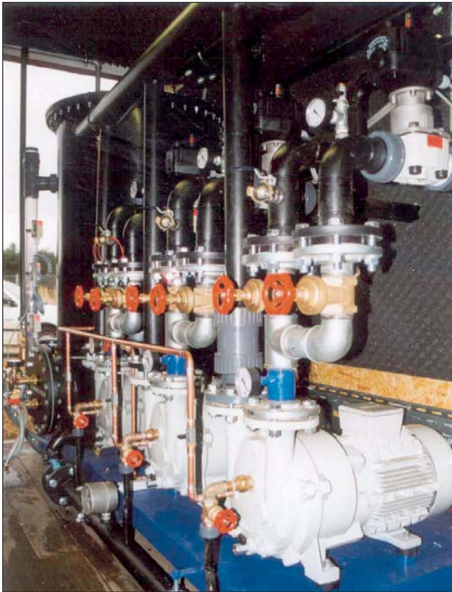
ATEX-conform water ring vacuum pumps for soil vapour extraction. Partial vacuum is produced directly at the wells.
