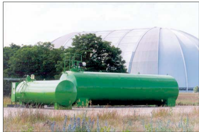
A 40m³ kerosene tank was used for collection of the recovered free phase. The kerosene was then reutilised as energy source for the on site power sets.
