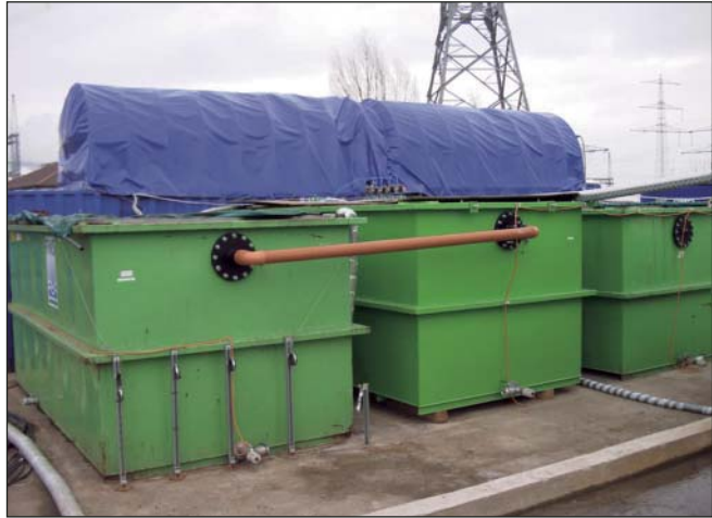
The treatment plant consists of coalescence separator, inclined tube settler, storage water basins and a tent-covered filter section with two sand and two activated carbon filters. It is appropriate for the treatment of 10 m 3 /h.
