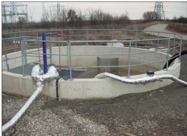
Apart from the groundwater treatment an additional 4 m 3 /h of surface water and construction site water has to be treated. As retention and sedimentation basin for the water serves a storage basin with a capacity of 70 m 3 .
