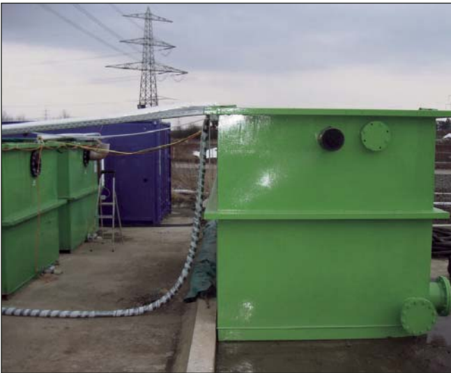
The sand filters of the treatment plant are backwashed time controlled respectively pressure controlled. The back washed sludge is buffered in the sludge storage tank (right) until its disposal later on.
