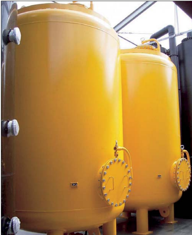
The last stage of the water purification consists of two liquid phase activated carbon filters connected in row. The purified water is afterwards infiltrated.
