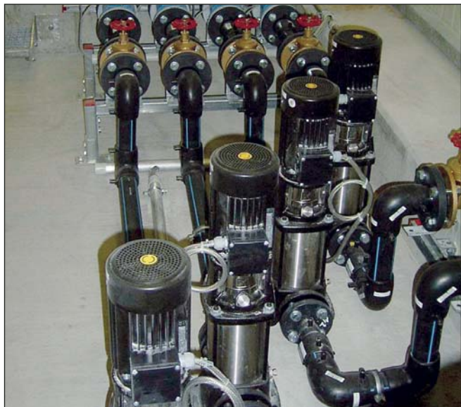
The pure water is infiltrated into the natural water regime in four infiltration wells. The individual wells are individually chargeable by pumps. The water flow is controlled by volumetric flow meter, which influences the quantity of water by valves.
