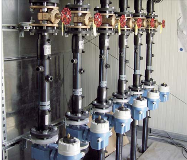
The water is pumped from six extraction wells. Each well is equipped with volumetric flow meter (magnetic inductive), manometer and throttling gates as well as a sampling valve.
