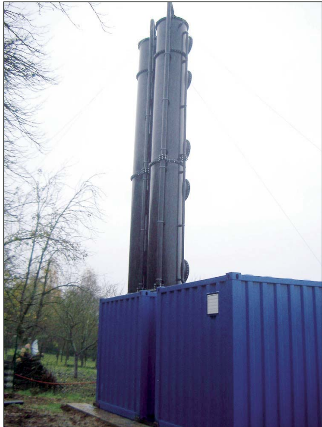
Two strippers, height 9 m (filling 6 m), one blower, one sand filter and a storage tank are placed in one of the 30 ft containers. The other container holds the backwashing system.
