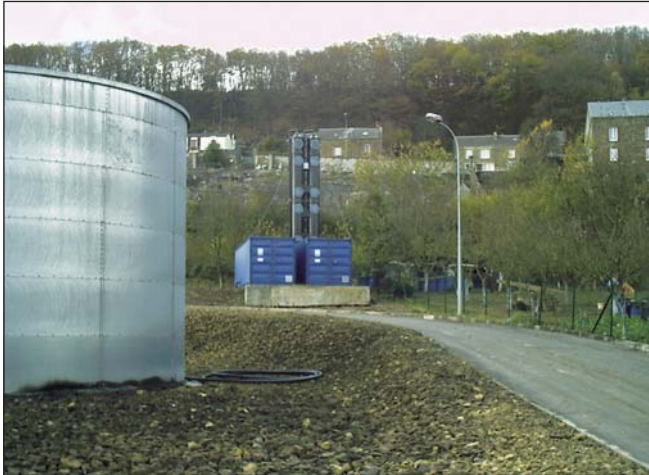
The treatment plant is installed in two 30 ft containers and the vacuum system is placed separately in a 10ft container.
