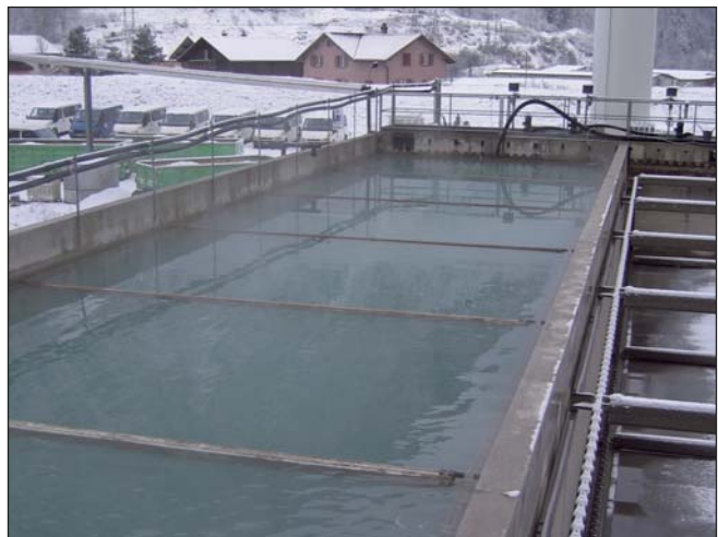
Treatment unit with circular scrapers for removing solids.
