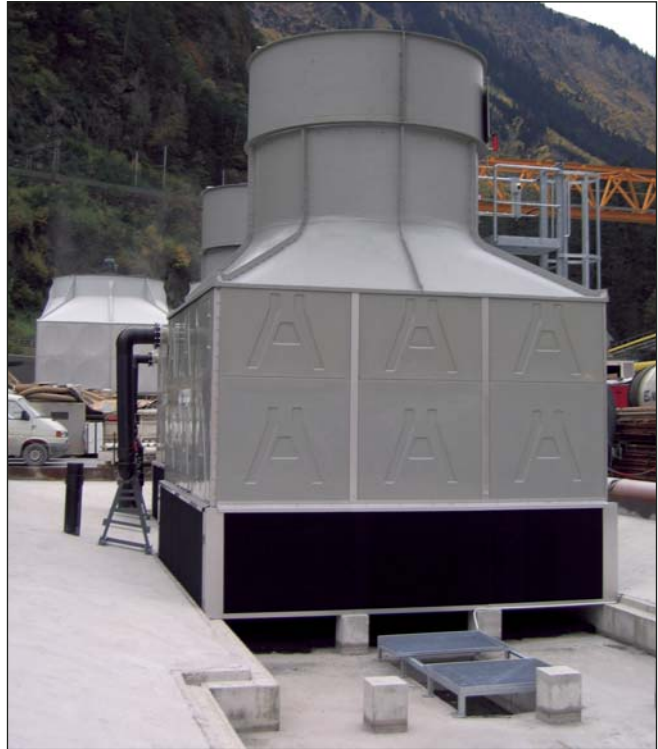
Sprinkling towers with special muffler in the standby mode.
