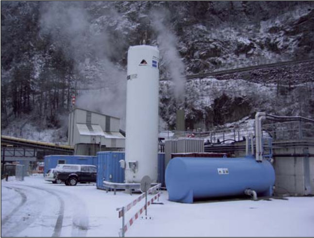
CO 2 -tank and process water container for the neutralisation of the treated water.
