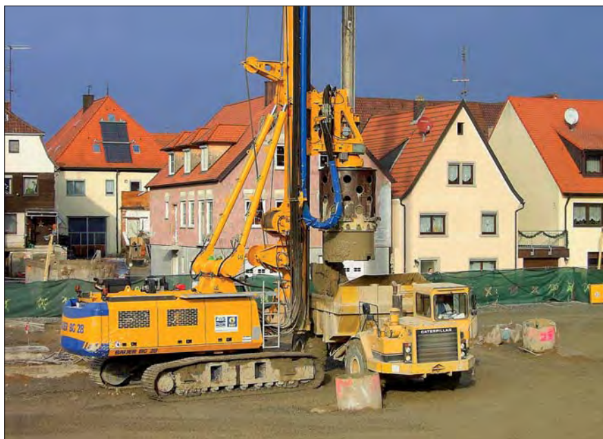
Due to the close vicinity of buildings and a complex hydraulic situation the contaminated soil was exchanged using replacement borings.
