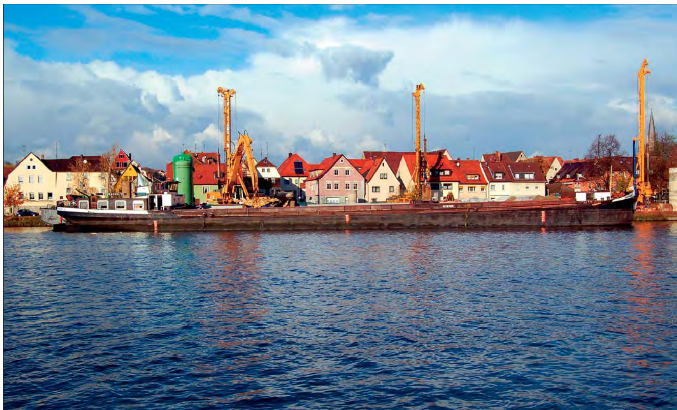
In order to avoid disturbance from heavy goods traffic, a shipping pier was erected to handle the transportation of construction equipment and contaminated material.
