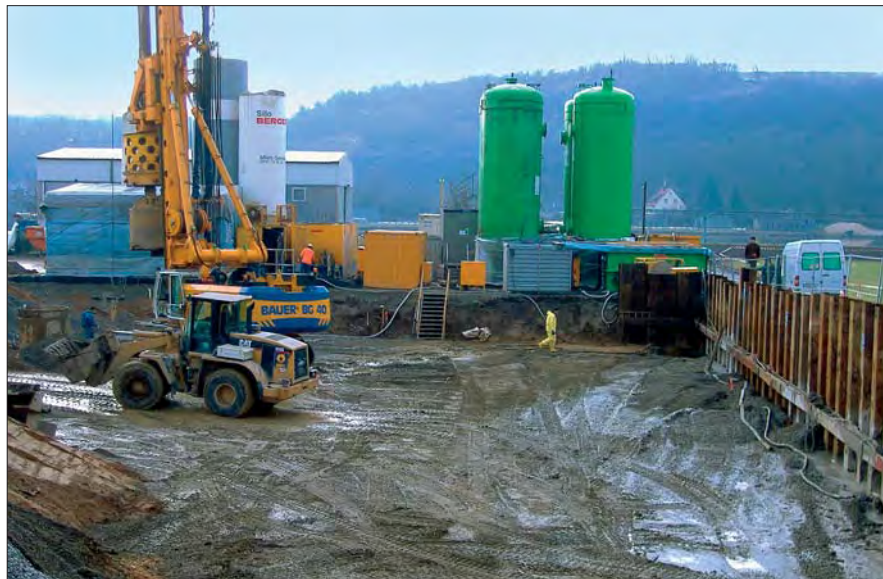
At the Schoberspitze site, the replacement borings were drilled from the level of a conventional excavation pit that was supported by a 500 m 2 sheet pile wall.
