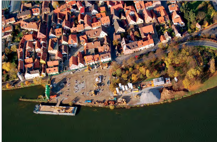
In order to complete the drilling operations before the expected winter flood, a second large diameter drilling rig was used at the Mainlaende site. Both rigs operated 6 days a week.
