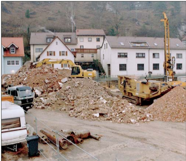
The mineral built volumes were broken on site and after an analytic investigation and the appropriate declaration, depending upon lead content, were either used for back filling or dumped.
