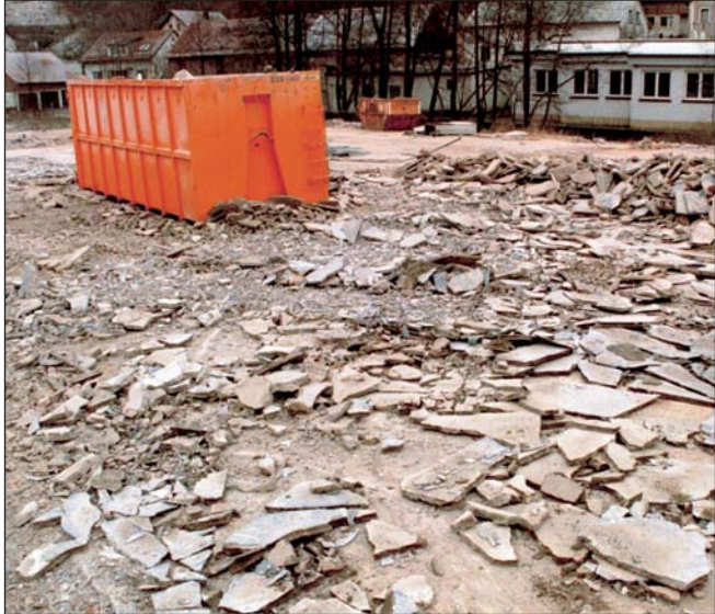
The screed loaded with petroleum-derived hydrocarbon was removed and the material was dumped on a disposal site afterwards.
