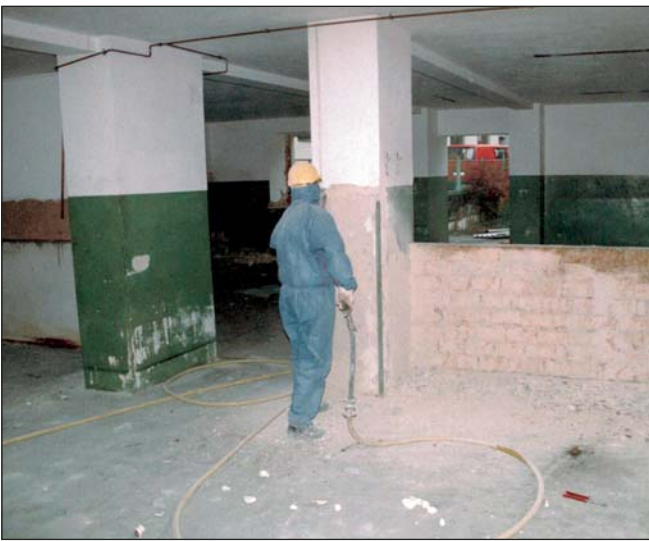
The existing buildings were cored before the deconstruction and hazardous and contaminated building materials were removed. Altogether 13,800 m 3 were backbuilt.
