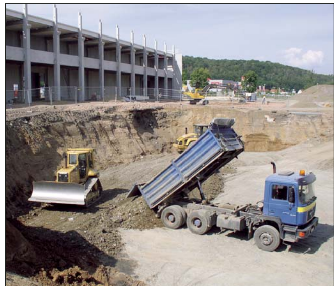
The backfill of the excavations took place in several layers with 112,000 to of non-contaminated material.
