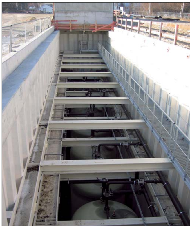
The central control panel, which monitors all parameters of the entire plant on-line, is located in gate 1. The gate is equipped with eight filter containers.
