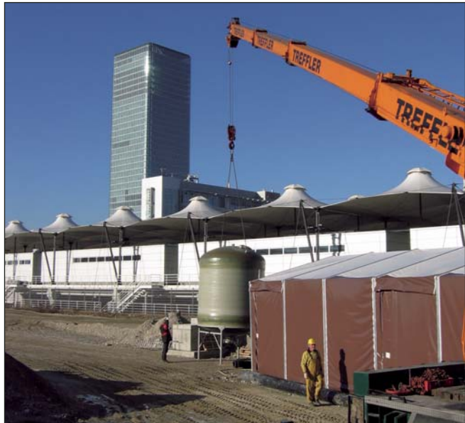
Installation of one of altogether 26 GFK containers for activated carbon (diameter 3 m) in one of the four gates. The base frame for the containers was made of V4A steel.
