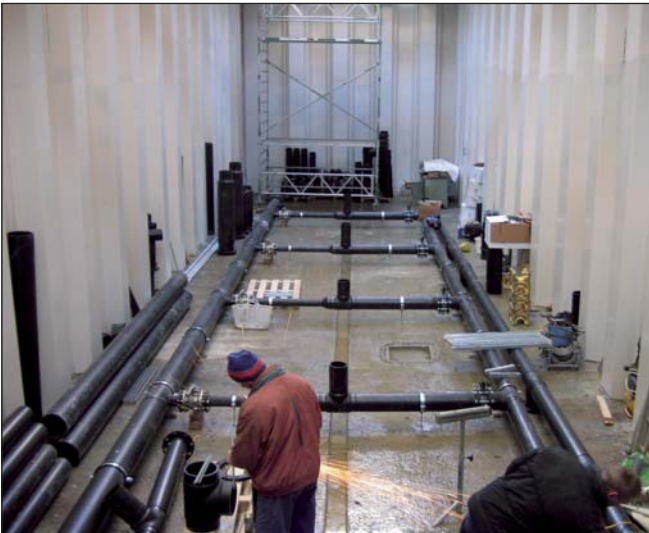
Inlet pipes and pipes for back washing were installed on site in the up to 35 m long gates. The gates are built as a steel sheet pile wall box.
