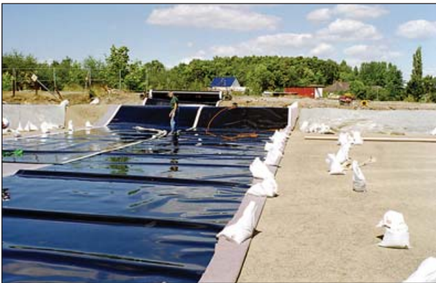
Construction of a "Mini landfill" on the site of the former smelting works with a fully sealed base for controlled and safe disposal of the contaminated residues from the original smelting process.
