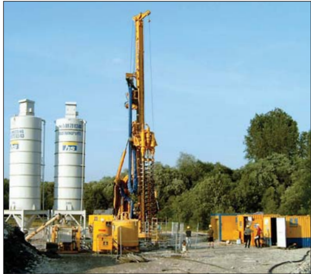
Plant and equipment used in the construction of a cut-off wall by the "Mixed-in-Place" technique patented by the BAUER Group
