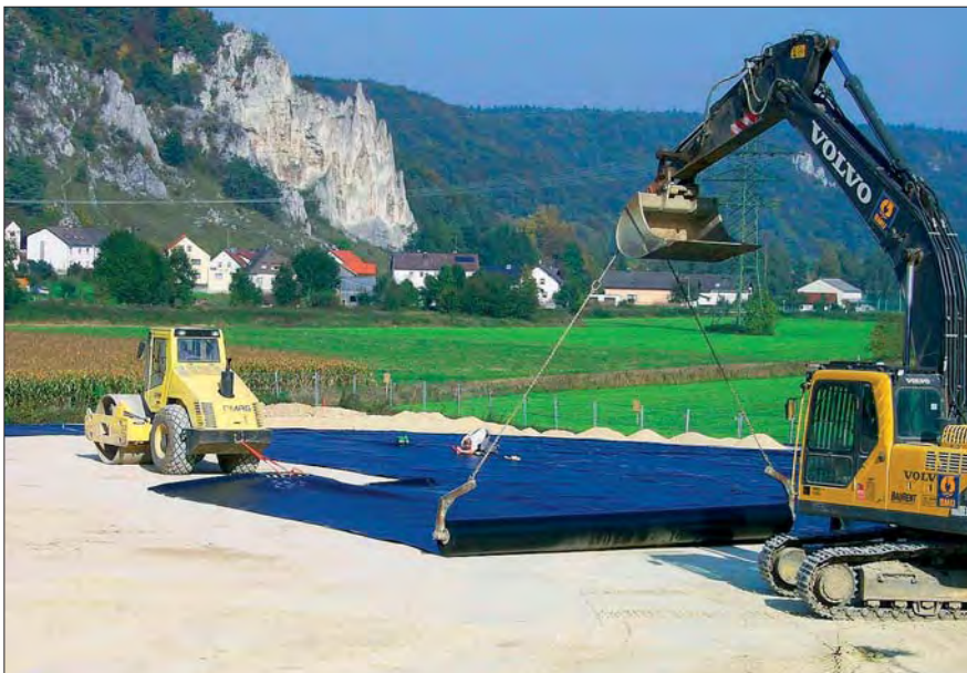
To secure the site against rainwater infiltration, a multi-layer cover system was constructed. Its base is a 2.5 mm thick HDPE sheet, the strips of which were sealed together and the joint then checked for leaks.
