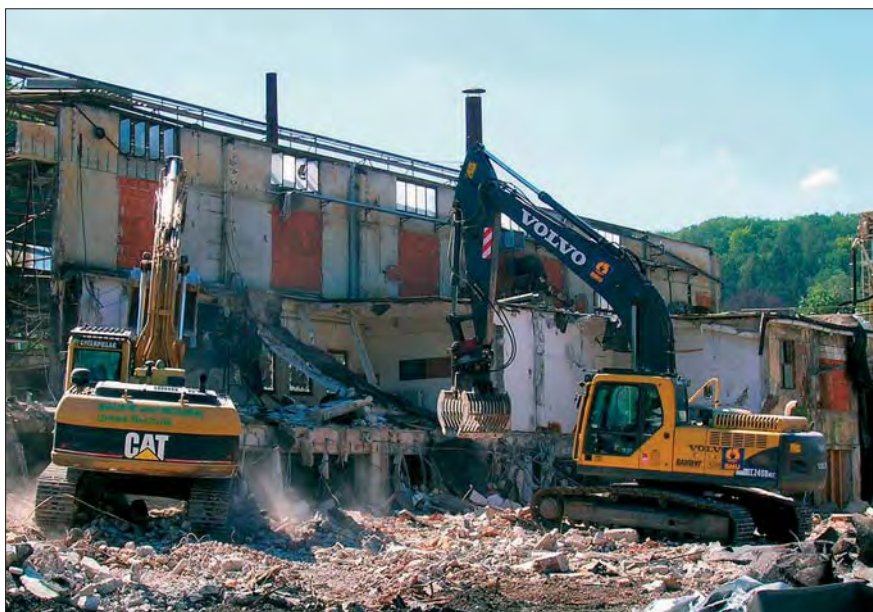
The demolition of the 22 blocks, some of which were as much as 12 metres tall, required the deployment of several excavators simultaneously.
