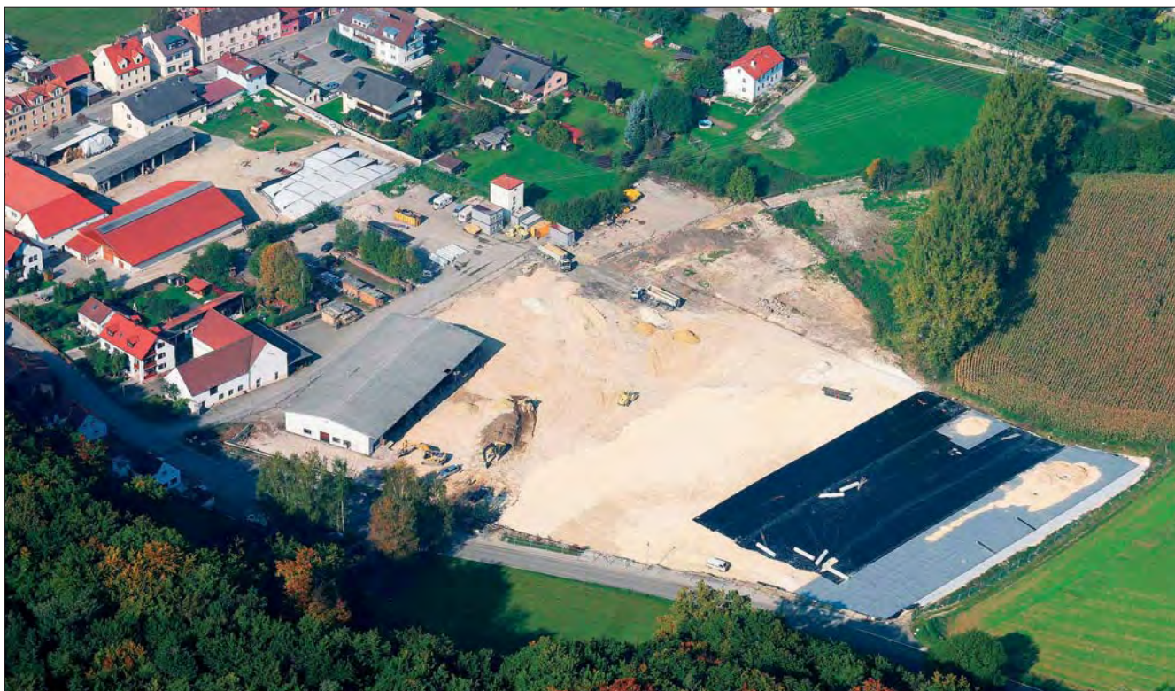
On the premises of the former Phoenix glassworks, a total of 22 buildings were taken down enclosing an interior space of 62.000 m 2 . The newly established surface was covered with a multi-layer capping system preventing rain water infiltration.
