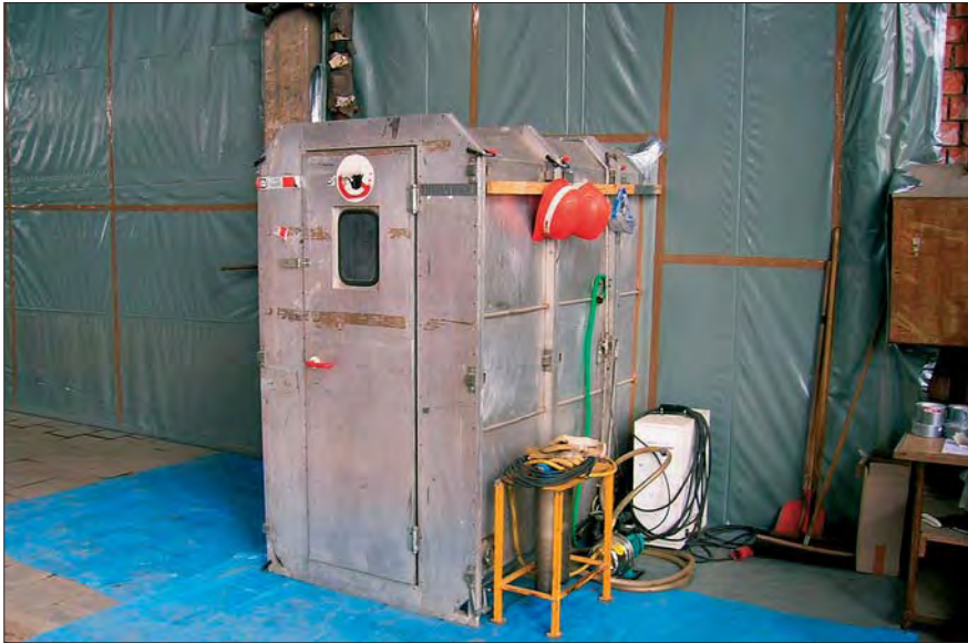
The air in the buildings was contaminated with asbestos, artificial mineral fibres and heavy metals. This required special occupational safety measures. Parts of the buildings were sealed off and made accessible only by way of a three-chamber airlock with a sub-atmospheric pressure system.
