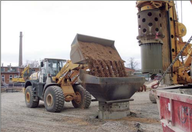
Boreholes were refilled after complete removal of the contaminated material with uncontaminated soil.
