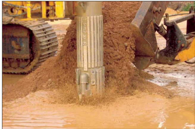
Due to high compaction requirements of the subsequent use of the site the remediated area had to be consolidated by vibrocompaction technology using a BAUER RG22/TR17.
