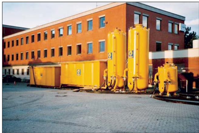
The groundwater treatment consisted of two sedimentation reservoirs, a sand filter, an activated carbon filter and a Cyanide treatment step.
