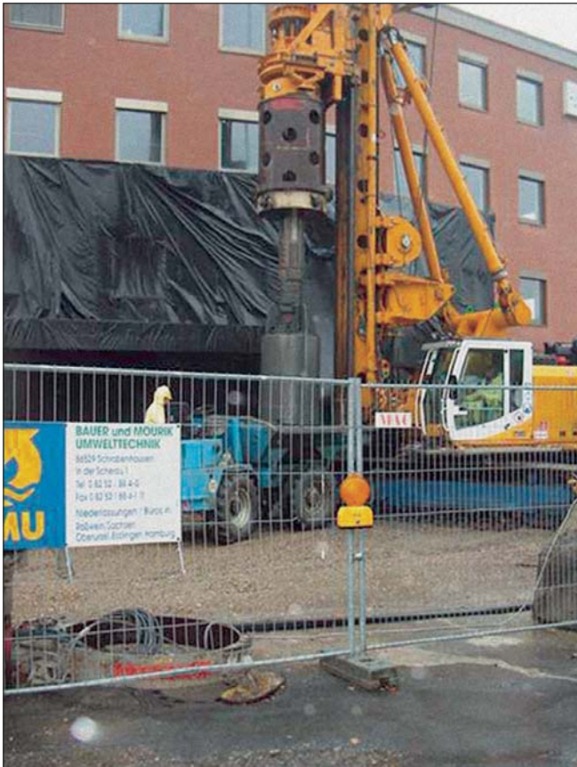
Contaminated soil is removed with a drilling bucket, then cement suspension and gravel is filled into the borehole.
