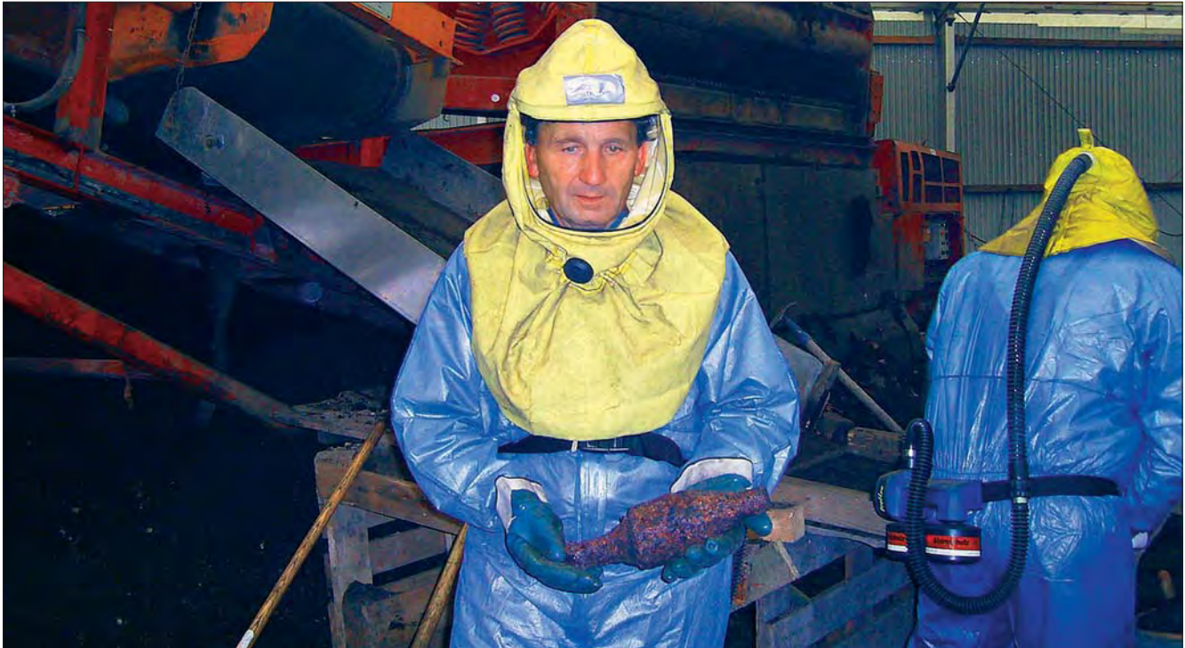
The munitions recovery placed high demands in terms of occupational health and safety. The personnel on site wore inherent protection suits and the wheel loader was equipped with a splinter shield.
