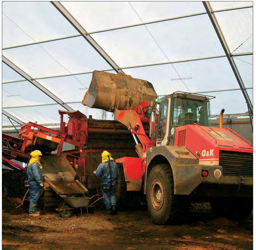
The heap material was sieved and a magnetic separator removed the ammunition remains. Subsequently, the soil was treated biologically in the soil treatment centre of BAUER Environment Group in Hirschfeld.
