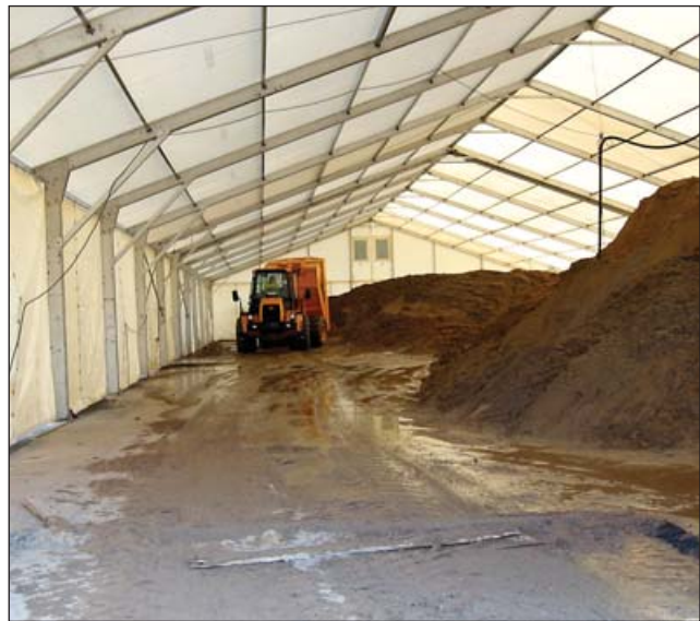
To prevent emissions escaping into the atmosphere, the excavated soil material was stockpiled in a tent prior to its removal off-site.
