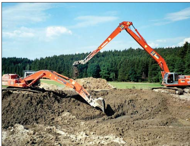
To excavate the polder basins a special excavator with a 15 m long boom was employed on site.
