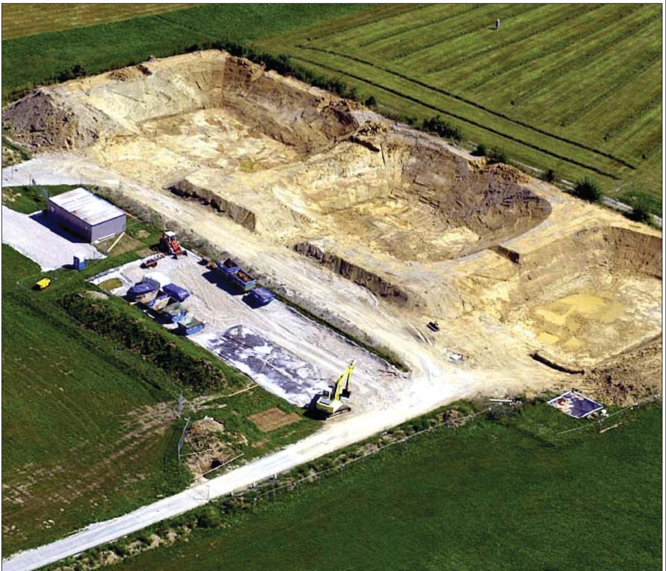
Drilling mud landfill site in Arlesried after excavation of the contaminated material.
