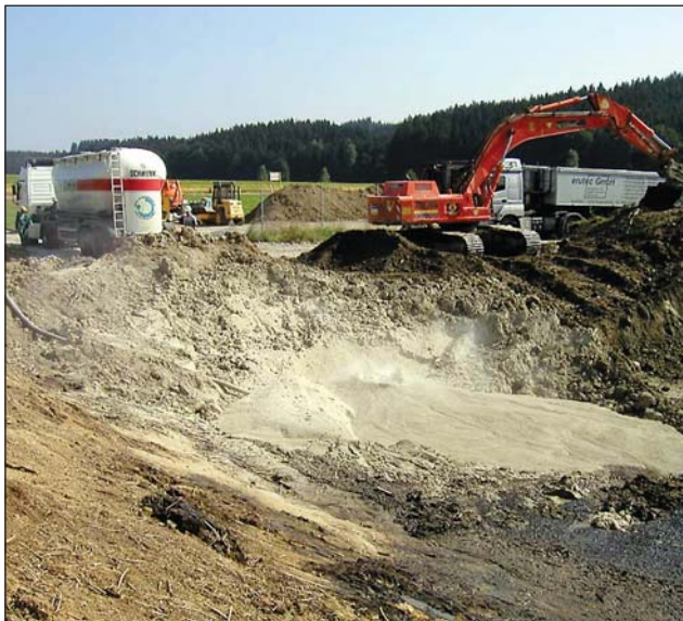
In order to make the excavated material suitable for transport a binding agent was used.
