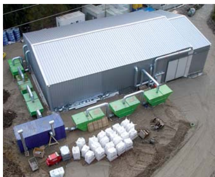
▲ Enclosure over the CLARK pit in Traunreut
