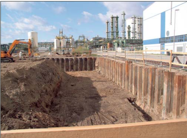
In order to protect the excavation pit from entering groundwater, it was enclosed with a 13 m deep sheet pile wall.
