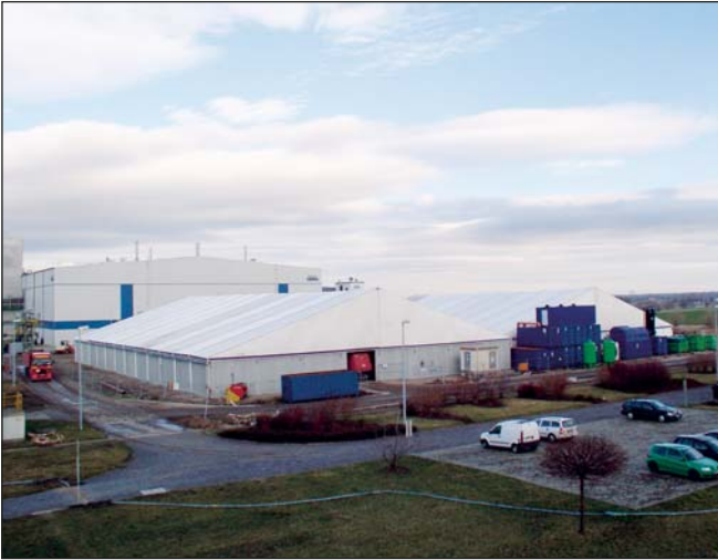
The building site, with excavation and supply camp, comprises approximately 6,000 m 2 was completely enclosed with two cantilever tents (90 m x 40 m and 60 m x 40 m).
