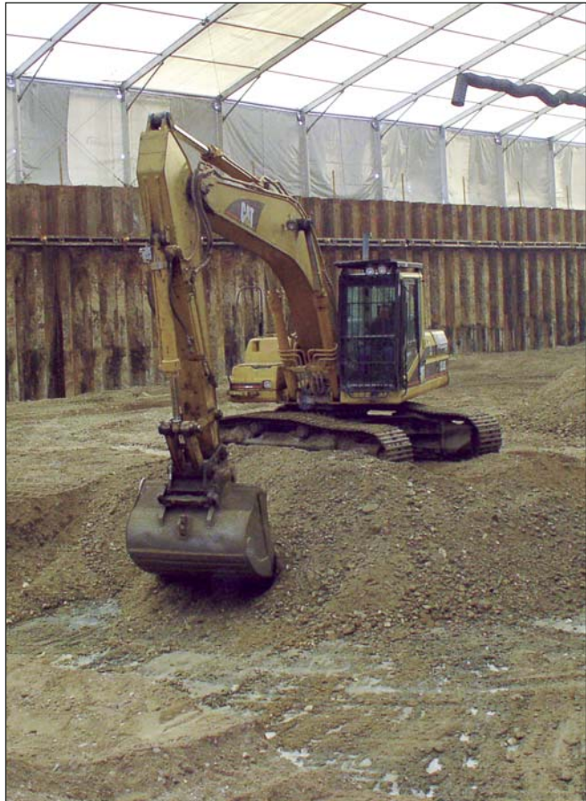
Due to the pollutant-enriched and highly combustible atmosphere a high performance ventilation system had to be used. The cleaning equipment was appropriate for volumes of 90,000 m 3 /h for the off gas and 20 m 3 /h for the groundwater.
