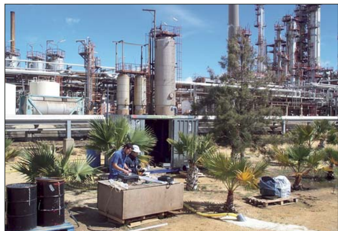
Vacuum compressors and waste gas stream cleaners are ATEX-conform and installed in a certified climate conditioned container.
