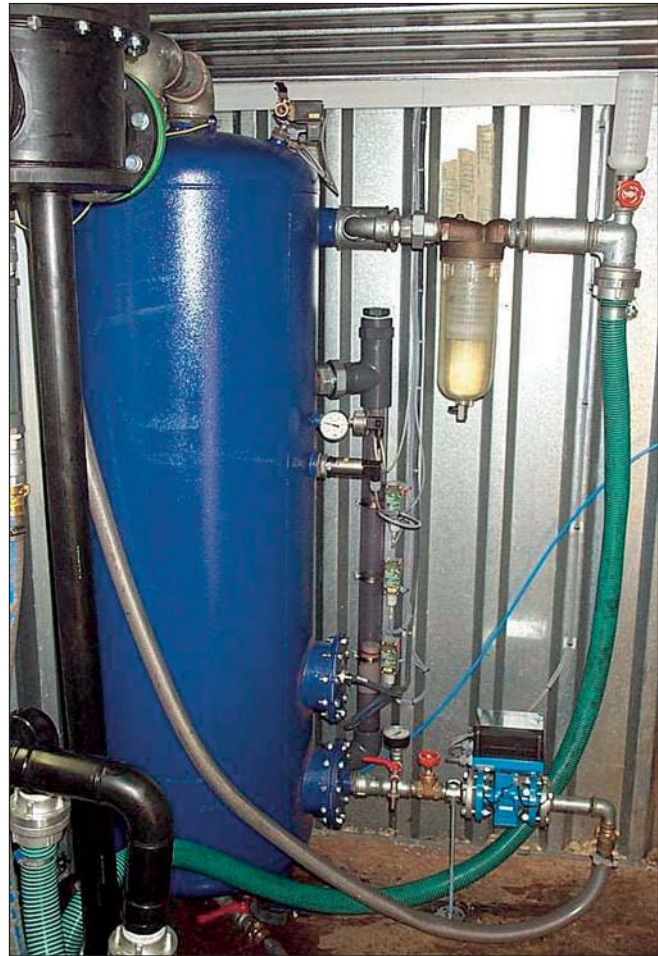
The contaminated groundwater is collected in a separator and is then automatically pumped through and treated by a liquid phase activated carbon stage. The storage tank for the non aqueous phase is equipped with a level switch, thus the plant is automatically shut down in case of overflow.
