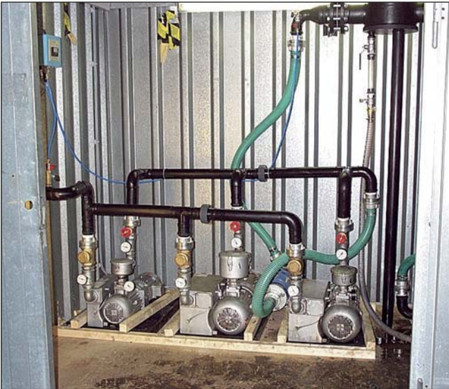
The FWS remediation plant basically consists of ATEX-conform vacuum pumps, bioslurping lances and vapour phase activated carbon filters.
