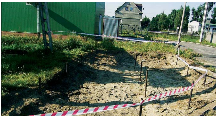
A mini excavator was used to excavate the heavily contaminated top soil. Thus, the efficiency of the remediation increased significantly.
