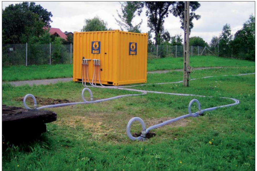
For the in situ remediation multiple wells were installed providing the soil with fresh air. Aeration and nutrients supply stimulate the activity of naturally occurring microorganisms which degrade the organic contaminants.
