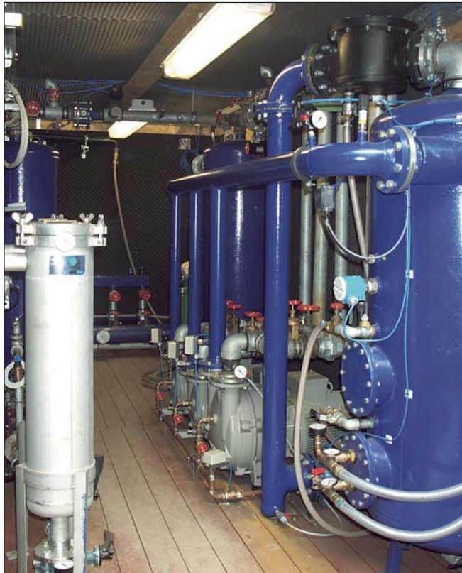
Several water ring vacuum pumps in different sizes allow an exact adjustment to the demanded suction capacity in the high and low vacuum range.
