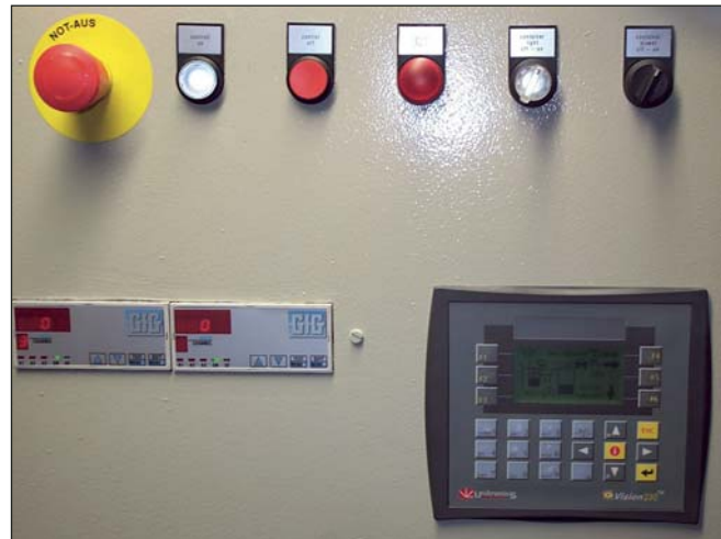
The entire control panel is accommodated in a separate container. Thus expenditure for the explosion protection was substantially reduced.
